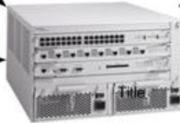
Nortel Networks ERS 8600 (Primary Switch)
